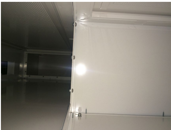
Modules Bolted Together
